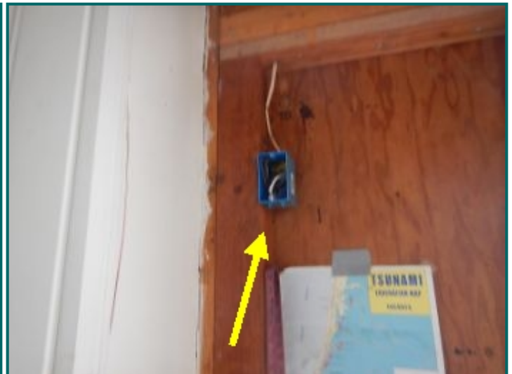
Electrical cover missing.
