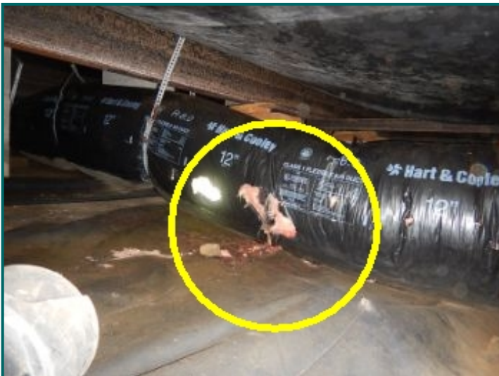
Ducting insulation damaged.
