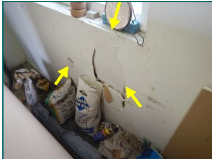
Dry wall damage noted.
