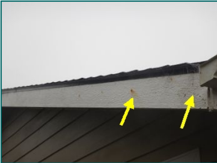
Water damage noted.
