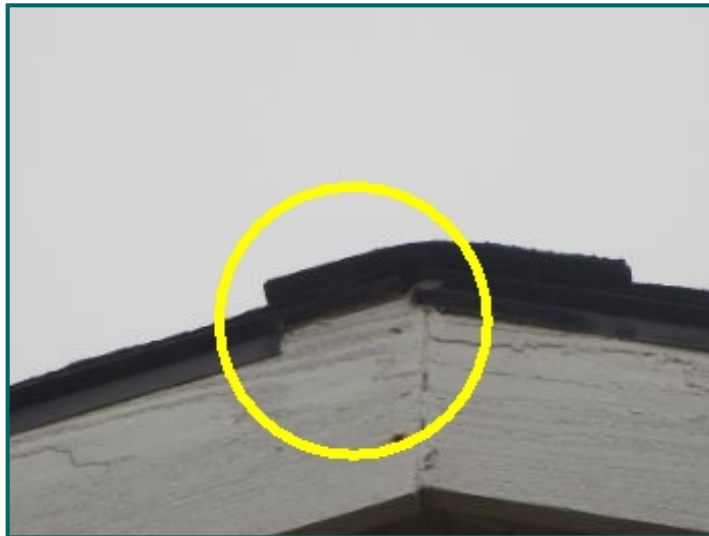
Incomplete drip-edge flashing
