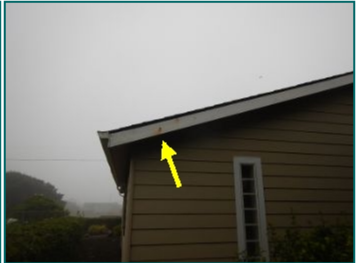
Water damage noted.
